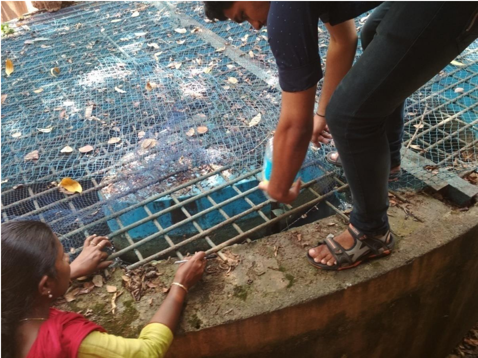
Chlorinating water tank
